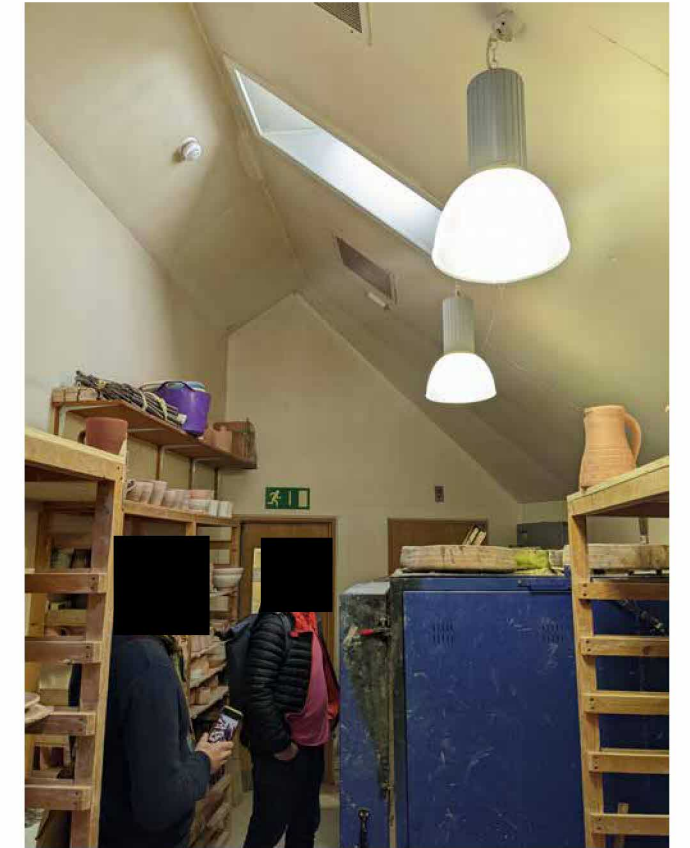
The production studio electric kiln room
